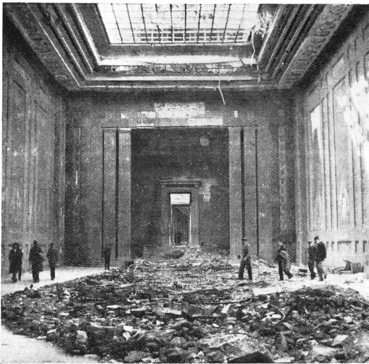
Inside the gutted Reich Chancellery, the floors of which abound in rubble. Adjoining rooms suffered even worse damage.
