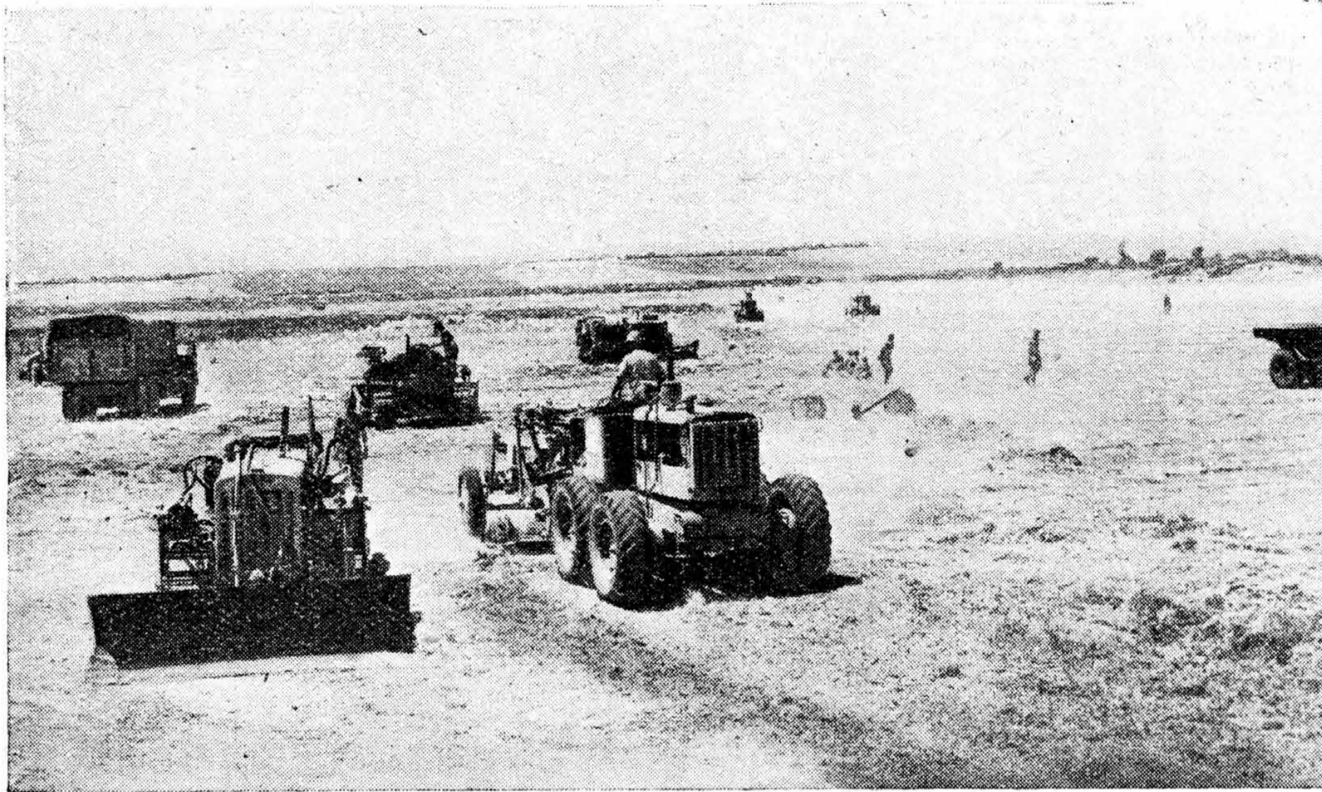
PLANING THE LAND.—A cornfield in Sicily, just harvested, is cleared and levelled for use as an Allied advanced landing ground.
