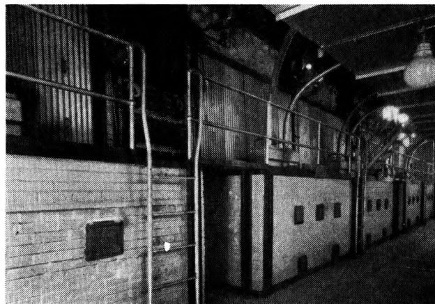
FIG. 1 HISTORIC PULVERIZED-FUEL BOILERS (Tests of boiler No. 5, in foreground, were subject of Bureau of Mines Bulletin. 2 )
