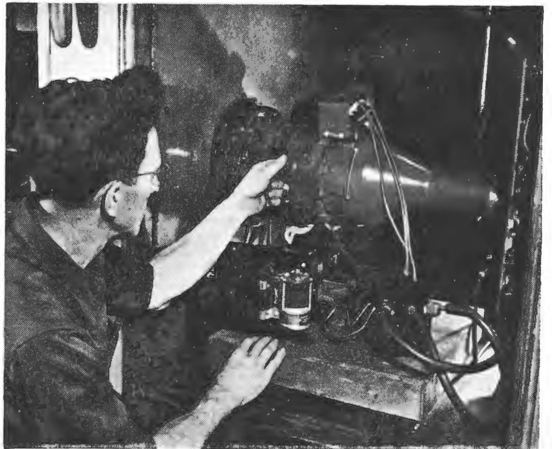
FIG. 5.—A 40-kva. alternator installed for an altitude-chamber test. The voltage regulator is being adjusted by the tester. To the right of the regulator is a three-phase 208/120-volt circuit breaker with a latched-in contactor
