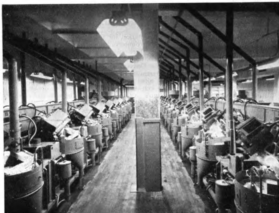
There are 32 Units in this installation used for sorting beans electronically.
